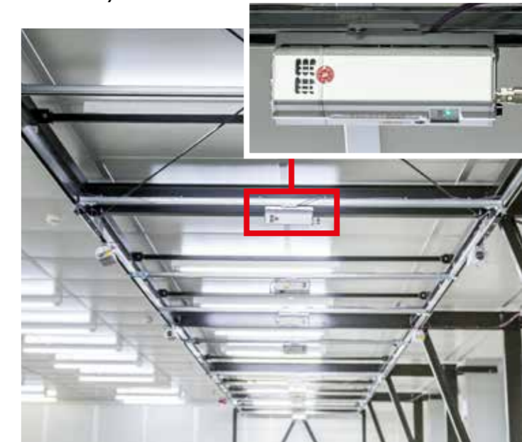
LAP CAD-PRO laser projectors are installed under the ceiling above the workstations. The system’s configuration is highly flexible, enabling it to handle tools of different sizes, which are positioned in the projection area on mobile tables.
